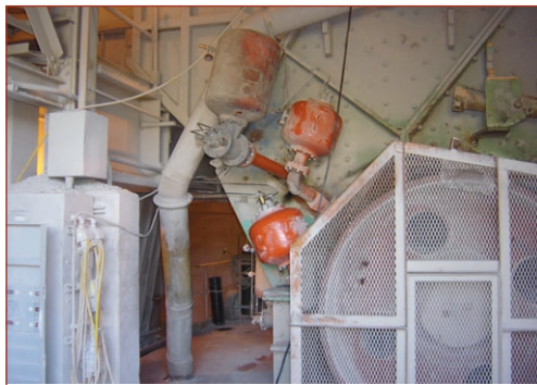
Figure 1. BIG BLASTER® XHV TORNADO (left) and HURRICANE Air Canons (two on right) installed on a cement plant's primary crusher.
