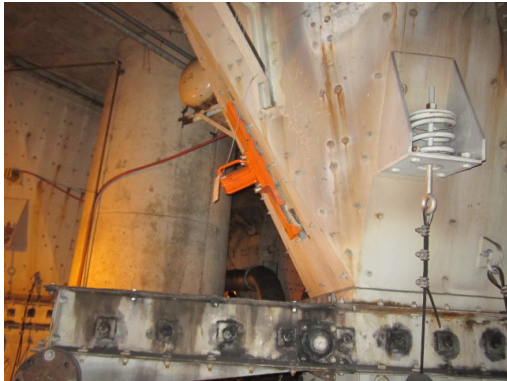
Cougar® Pnuematic Piston Vibrators installed on a hopper at the Bonanza Power Plant in Vernal, Utah.
