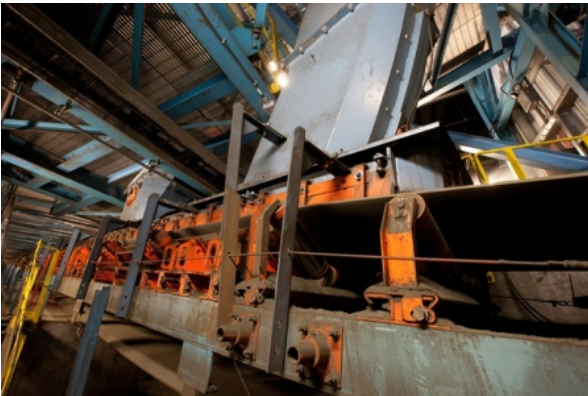
The new transfer points employ a "hood and spoon" transfer to place material onto the belt being loaded.
