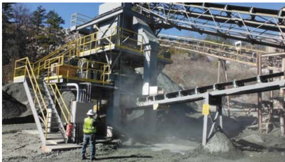
BEFORE: Loader operators used the cloud of dust to determine if the crusher was working properly.
