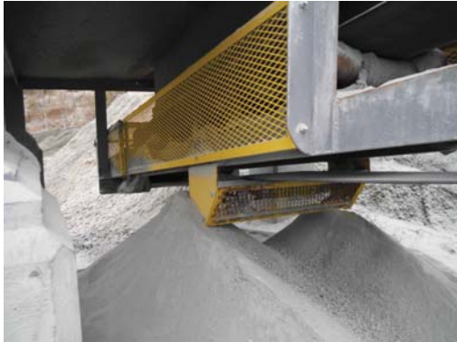
Before Martin Engineering's transfer point upgrade, the plant encountered significant spillage.
