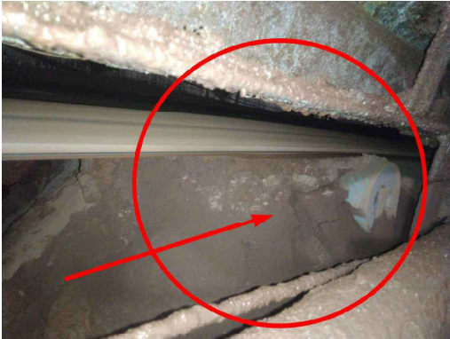
Once encapsulated, the roller seized and wore on one side, causing friction heat and a potential fire hazard.
