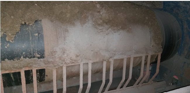
Previous cleaners allowed carryback to remain due to inadequate tensioning and uneven contact.
