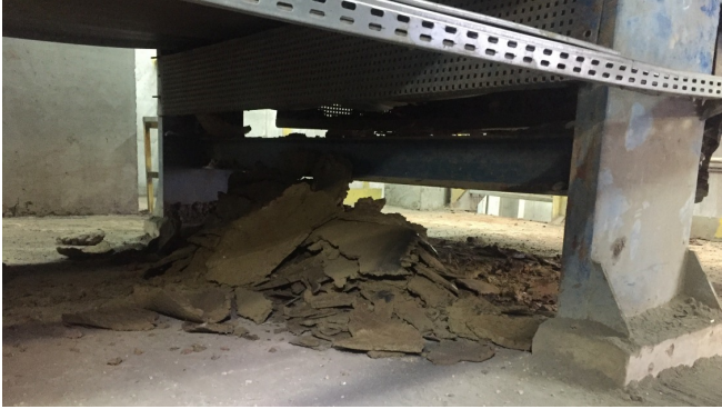
The curve of the head pulley caused the carryback to crack and drop below the belt in sheets.
