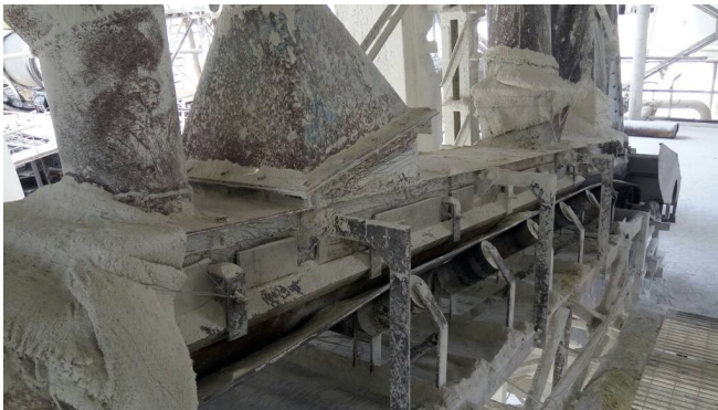
Material loss, potential health & safety hazards and excessive cleanup time were all motivating factors.
