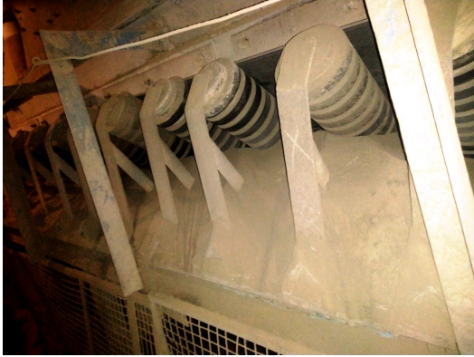
Skirtboard seals fabricated in-house using old rubber belt were causing belt damage, spillage and dust.
