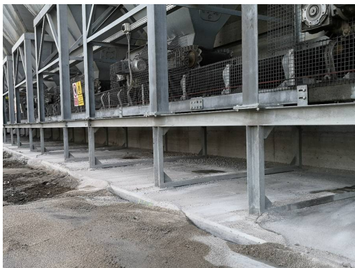
Daily cleanup of spillage has now been reduced to removal as needed just once every 6-7 weeks.
