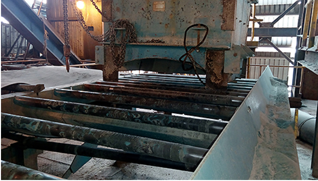
The high impact bent rollers and damaged bearings, increasing downtime and maintenance costs.
