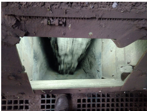
More material is discharged into the chute with no buildup and no manual cleaning
