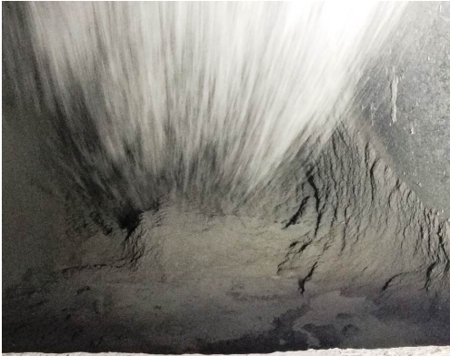
Substantial buildup was being observed on conveyor discharge chute wall, requiring periodic manual cleaning
