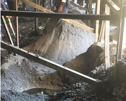
Piling waist high in some places, the spillage extended onto walkways and restricted safe access.
