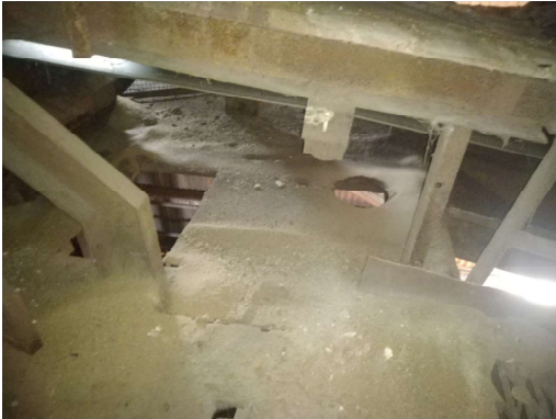
Ineffective belt cleaning led to extensive carryback, which accumulated all along the return run.
