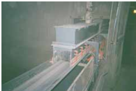
The transfer point reconstruction project included installation of new chute walls, covers and dust curtains on all three conveyors.
