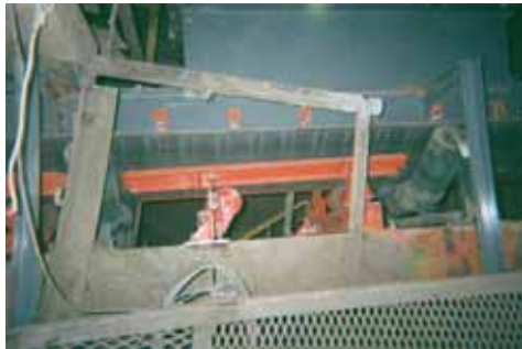
To stabilize the belt path, each load zone now includes Martin® Support Cradles with stainless steel bars for high temperature applications.
