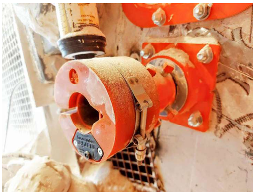
The N2 Position Indicator works with belt cleaners to maximize service and inspection efficiency.
