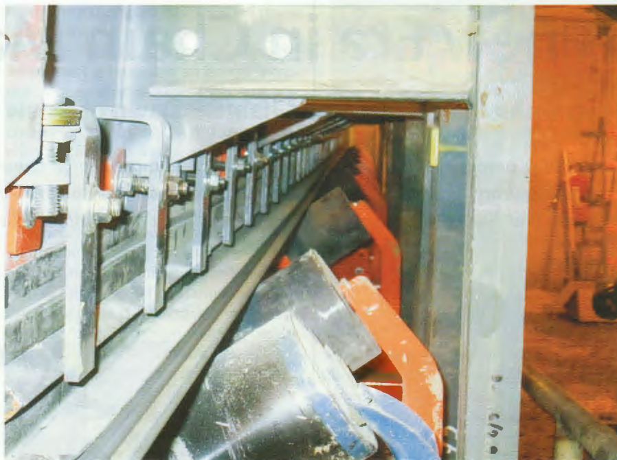
The external skirting system seals the chute to the belt.
