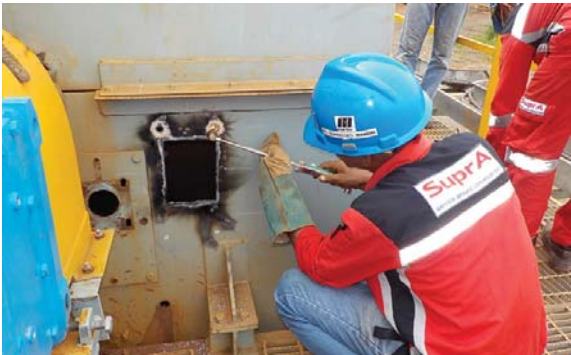
Technicians examined the issue and installed a Martin® QC1™ Cleaner HD and Martin® DT2 Inline Cleaner.
