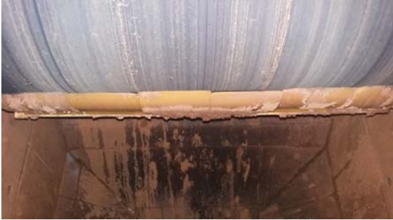
Rocks would wedge in the primary belt cleaner, breaking the splice and shredding the belt.
