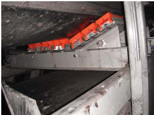
Martin Engineering installed Martin® Impact Cradles on the Enertec conveyor belt used to recycle car batteries.
