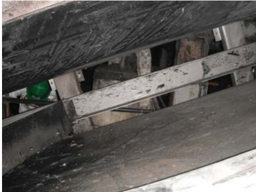
Enertec's conveyor belt suffered from impact damage and misalignment..
