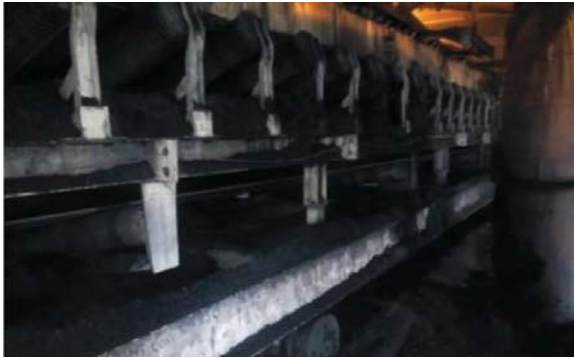
Adani Power Maharashtra in Gondia, India was experiencing problems with dust, spillage and carryback.
