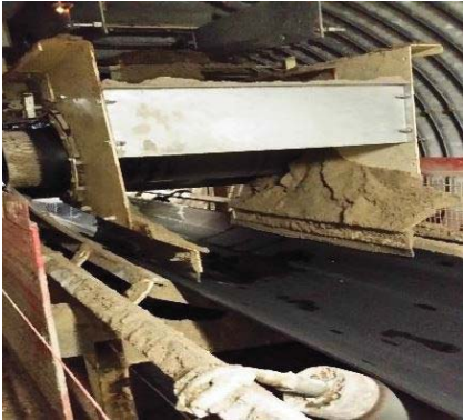
A cement plant on a site in the Rhône, was experiencing excessive spillage from one of its conveyor belts.
