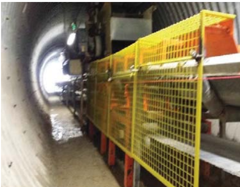
Martin® Conveyor Guards were added to protect workers from conveyor nip points and pinch point hazards.
