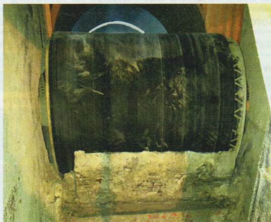
6 The prior blade got encrusted with material, degrading performance and accumulating build-up
