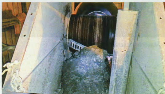
8 The increased flow of material cleared from the belt required a vibrating dribble chute to be installed
