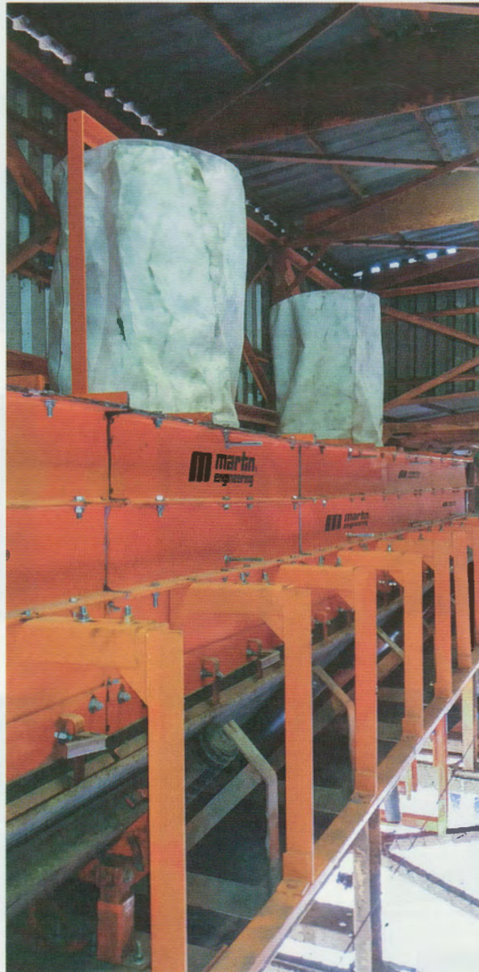
5 The new loading zone featured a sealing system that mitigated spillage and dust supported by dust bags
