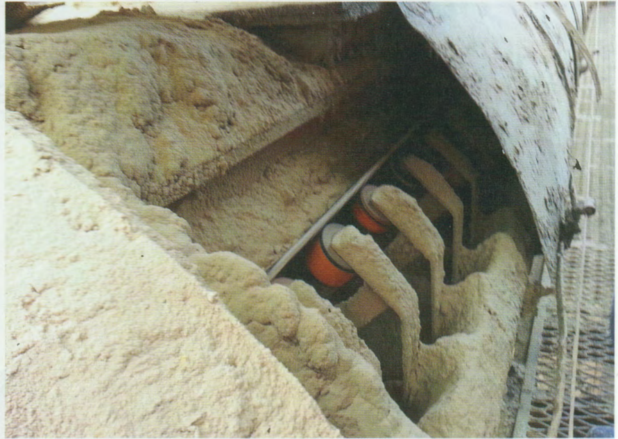
4 Dust and spillage clogs idlers, requiring them to be replaced and raising the cost of operation
