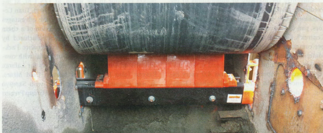
4 At PVDC, Martin Engineering replaced primary and secondary belt cleaners at 16 discharge points
