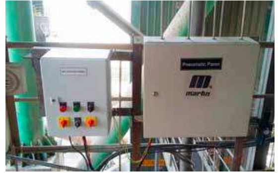
6 A solenoid box located far from heat and danger areas provides easy access
