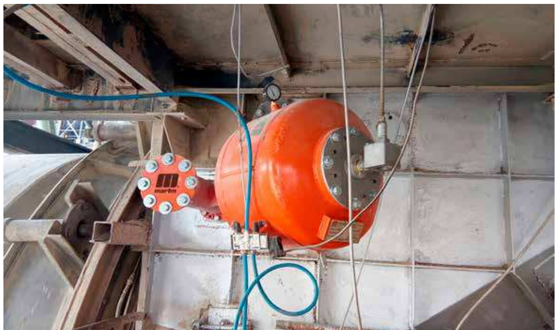
7 The outward facing valve allows safe servicing by one worker, without a shutdown
