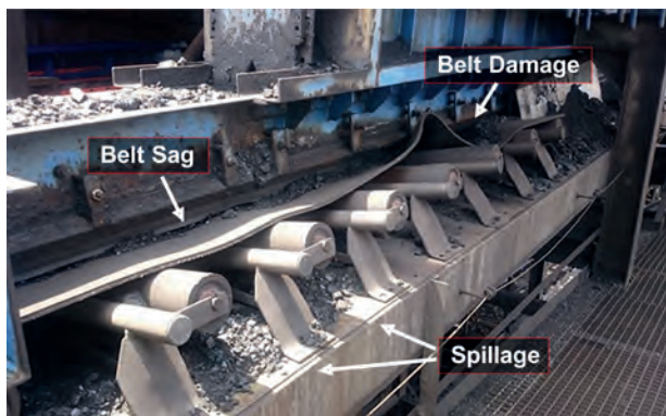
Figure 4. Broken equipment, spillage, and improper idler spacing all culminated in expensive consequences.
