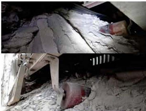
Figure 8. The roller is encapsulated by spillage at the discharge zone.
