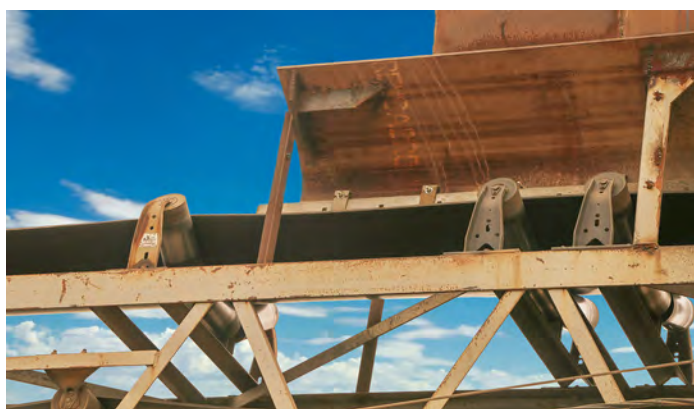
Figure 1. This an example of a fabricated curved skirtboard, which are hard to maintain when replacing wear liners and skirting.
