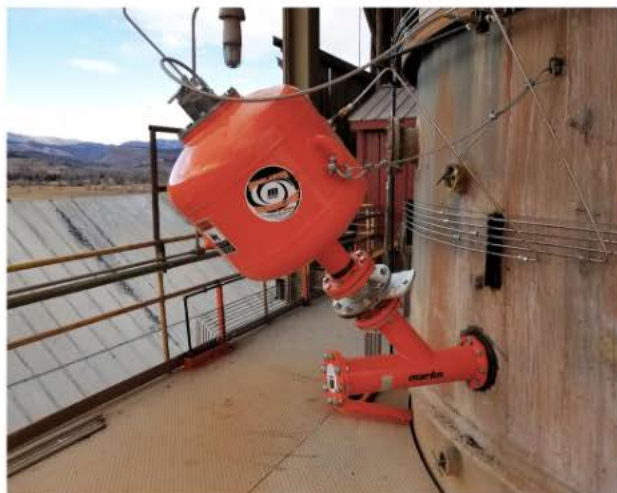
The outward facing valve allows safe servicing by one worker, without a shutdown.
