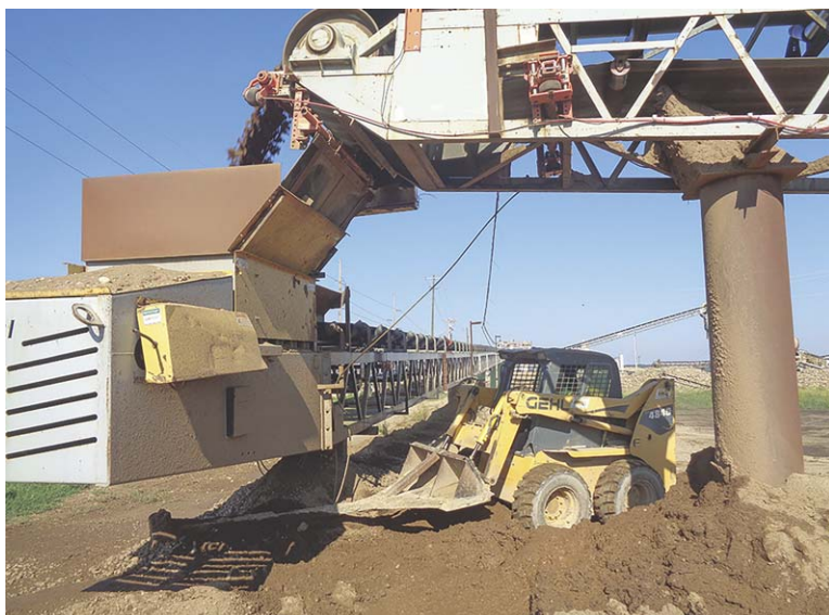
Figure 8. Cleanup under a conveyor can divert essential staff from more productive tasks.
