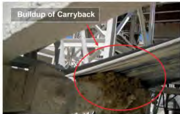
Figure 2. Inadequate cleaning leads to carryback build up and potential encapsulation.
