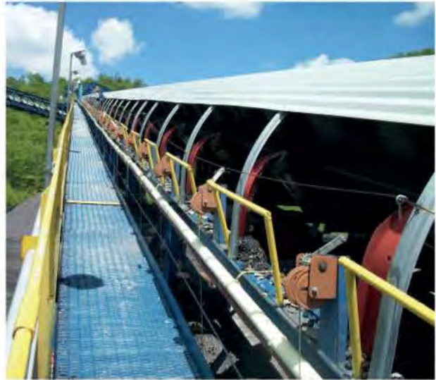
Figure 4. Hinged drip pans designed to be lowered with winches.
