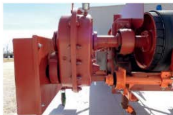
Conveyor drive motors can be as large as 600 HP (450 kW), moving belts as fast as 2000 ft/min. (10 m/s).
