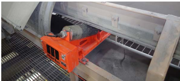
The outside diameter of the generator matches that of the roll, but places the unit outside the material path.
