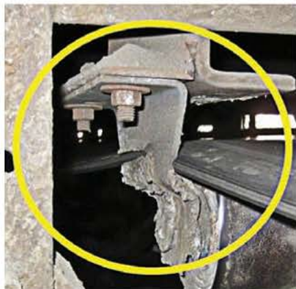
Belt mistracking is a common indicator that maintenance is due.
