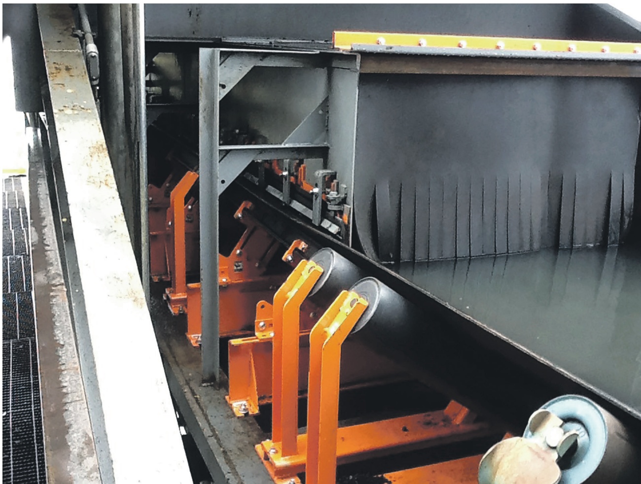
An effective transfer point requires the belt's line of travel to be stabilized and supported.
