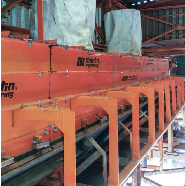
The new loading zone featured a sealing system that mitigated spillage and dust supported by dust bags.
