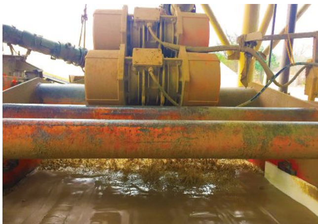
The wet slurry jumps across the screen as moisture drains through the fine mesh cloth.
