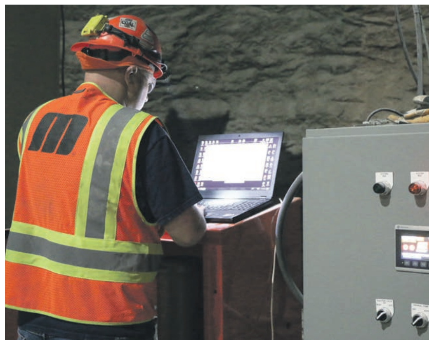
Integrating the system with the plant's PLC helps operators to monitor and adjust chemical outputs.
