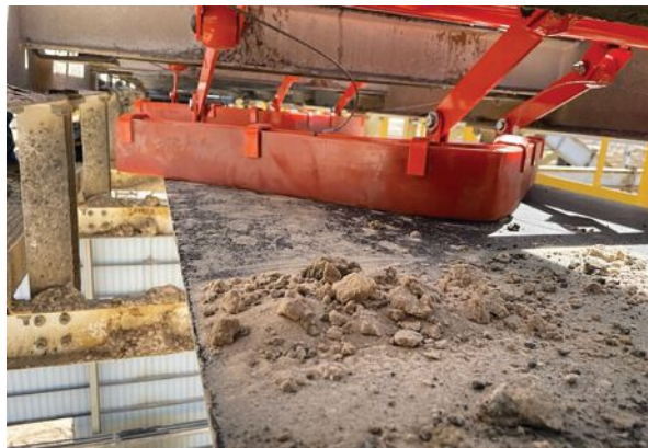
A plow diverts fugitive carryback to either side of the system, ensuring tail pulley health.
