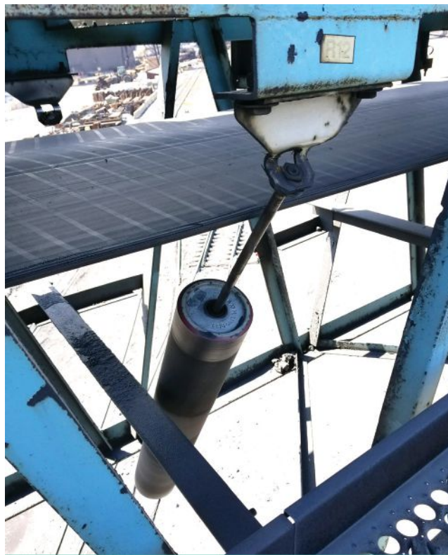
A run-till-it-breaks approach can introduce significant safety hazards. (Photo: ©Martin Engineering)
