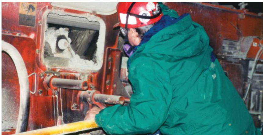
Detecting problems before they arise is at the core of PM and PdM. (Photo: ©Martin Engineering)
