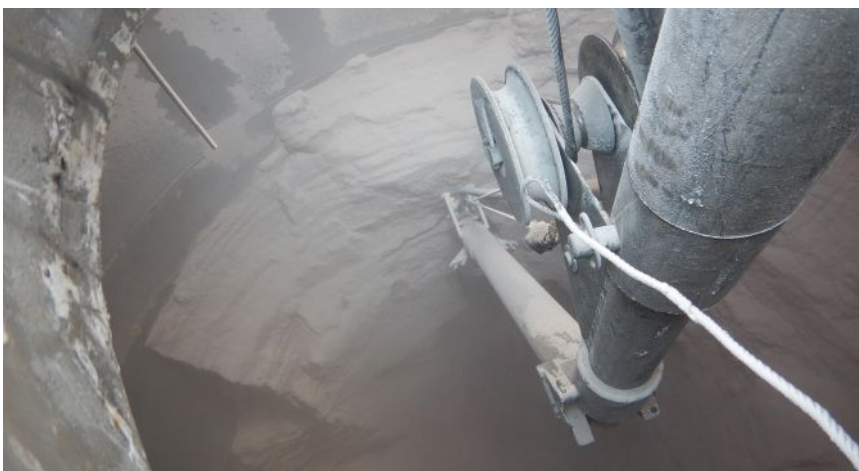
Lowered into the silo from the access hatch, the device operates from the bottom up.
