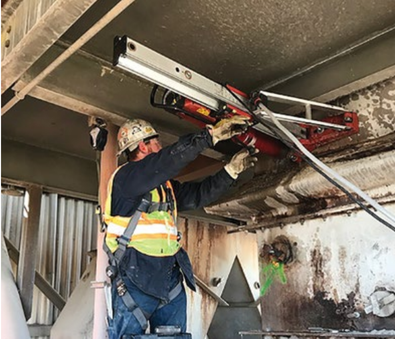
New technology allows air cannons to be installed and serviced without a process shutdown.
