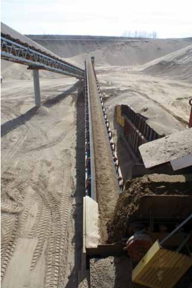
Changes in belt speeds or material properties can drastically impact the efficiency of a non-linear transfer point.
