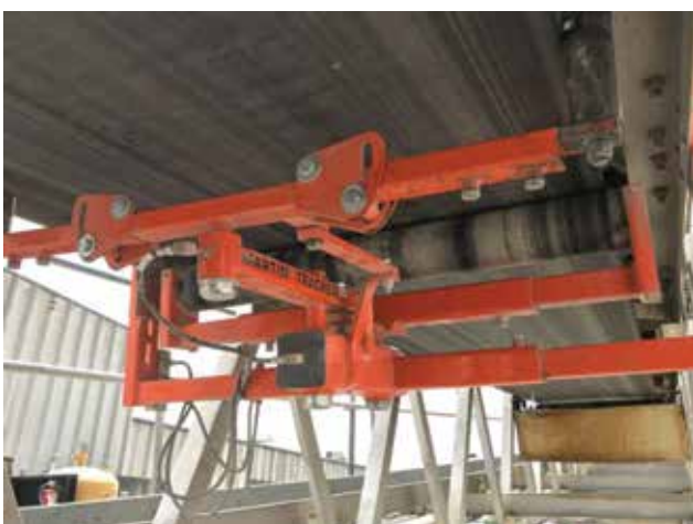
The return side Martin Tracker lifts the belt slightly for appropriate contact.
