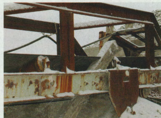
A wooden block used (unsuccessfully) to limit belt wander
