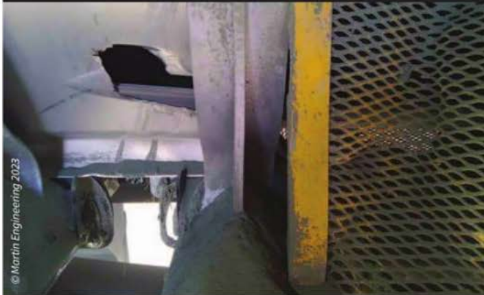
The large hole and the warped grate indicate the extreme heat emitted by the system
