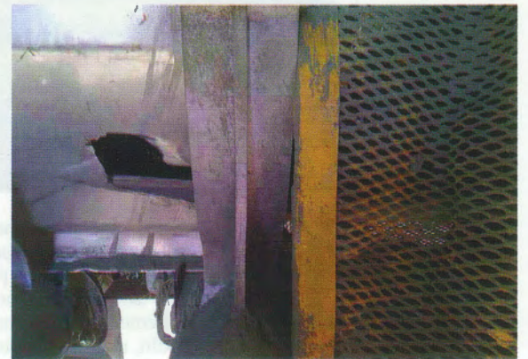
The large hole and the warped grate indicate the extreme heat emitted by the system
