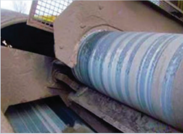
The existing metal blade delivered poor cleaning performance, while damaging the belt and splice. Copyright © 2023 Martin Engineering
