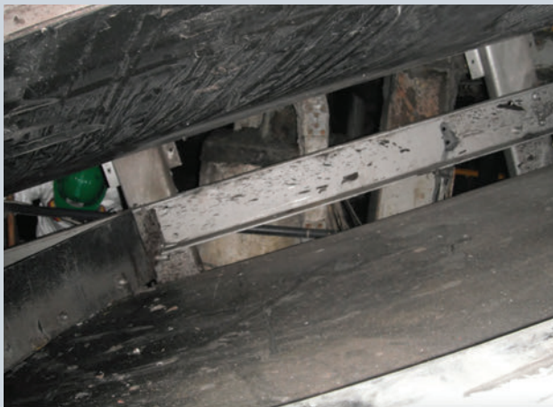
Enertec's conveyor belt suffered from impact damage and misalignment. Copyright © 2023 Martin Engineering
