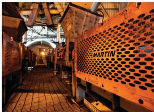
Figure 4. Conveyor guarding with the proper grating protects from flying spillage.
