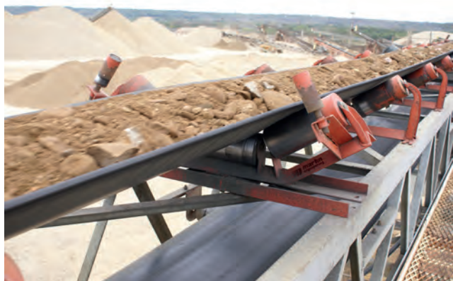
Figure 4. Belt tracking keeps loads centred and minimises dust from spillage and disruption.
