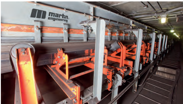
Figure 4. A cradle and idler system ensure a smooth and sealed belt path through the length of the chute.
